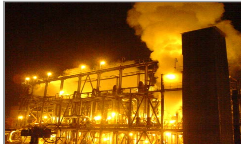
Night view of the security filtration
